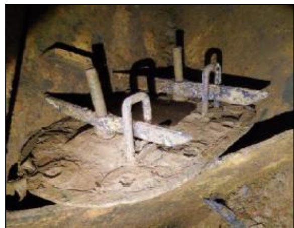
Figures 18-19: Manhole covers with wrongly fitted strong backs
