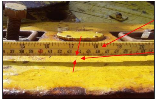
Figure 10: Deformation (set-down) of one of the manhole cover by about 4 to 5 mm
