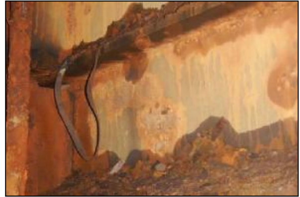
Figure 15: Another displaced rubber seal inside a ballast tank
