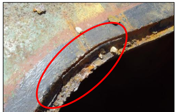
Figure 11: Corrosion on the sealing face
