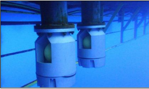
Figure 6: Vent pipes (capsized barge)
