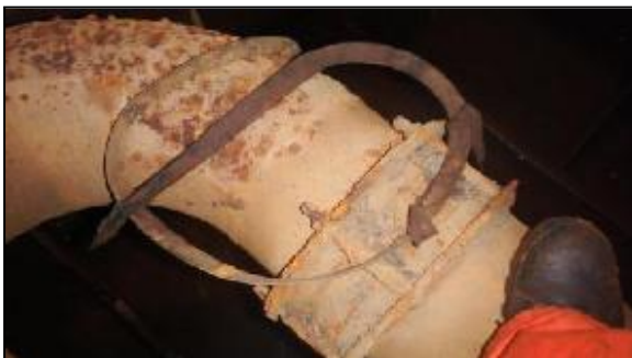
Figure 14: Displaced rubber seal inside a ballast tank
