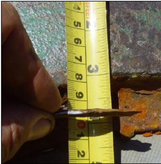
Figure 12: Flaking material due to corrosion, compromising a watertight arrangement
